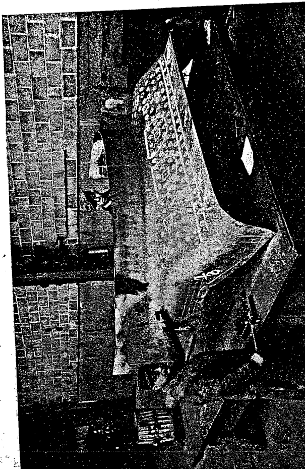
Laying out an outside throat sheet on the large surface block after flanging
