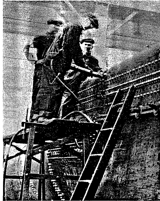
On receipt of the boiler, the odd rivets, which can not be fitted on the bull riveters, are driven by hand
