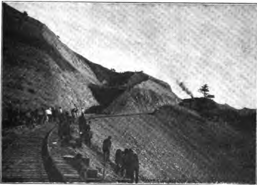
MOFFET ROAD TUNNEL CONSTRUCTION AND TEMPORARY TRACK AROUND IT.—F. J. FRANCIS, PHOT'R.
