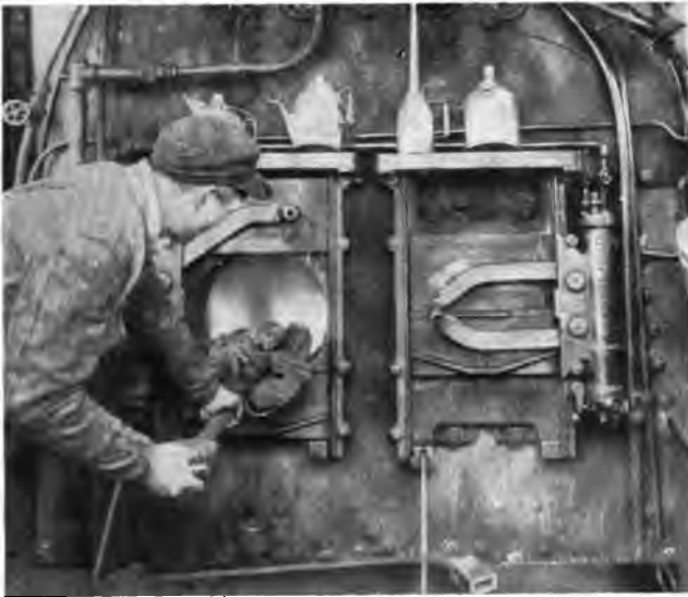
Fig. 332. Pneumatically Operated Vertical Fire Door. Open Position.
