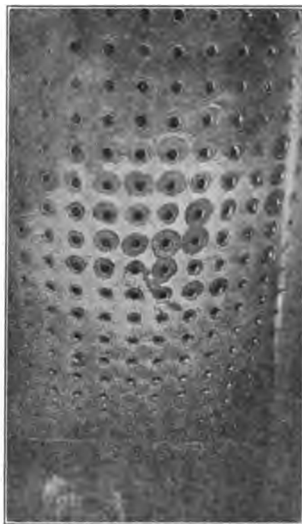
Fig. 1. Shows a crown-sheet failure, due to low water, which resulted in the injury of one person. The crown sheet was overheated its entire length and pulled away from 313 radial stays of the oil-burning type, which stays have hammered heads and are tapered on the fire box end 1/2 inches in 12 inches. All fire-box seams were riveted. The crown sheet pocketed to a depth of 16 1/2 inches. The tops of both the flue sheet and door sheet for a distance of 36 inches were bent downward to an angle of 45°.
