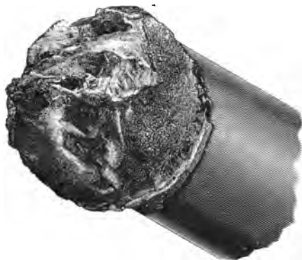
FIG. 1. — A FEED-PIPE NEARLY SEALED UP BY SCALE.
