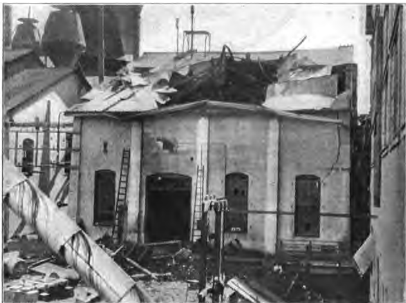
DAMAGE TO ENGINE HOUSE BUILT OF 12" CONCRETE WALLS.
