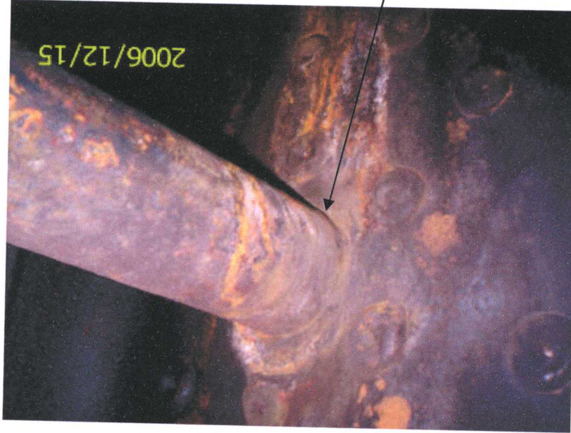
Photo 7. Leaking arch tube expansion (LH tube rear end)
