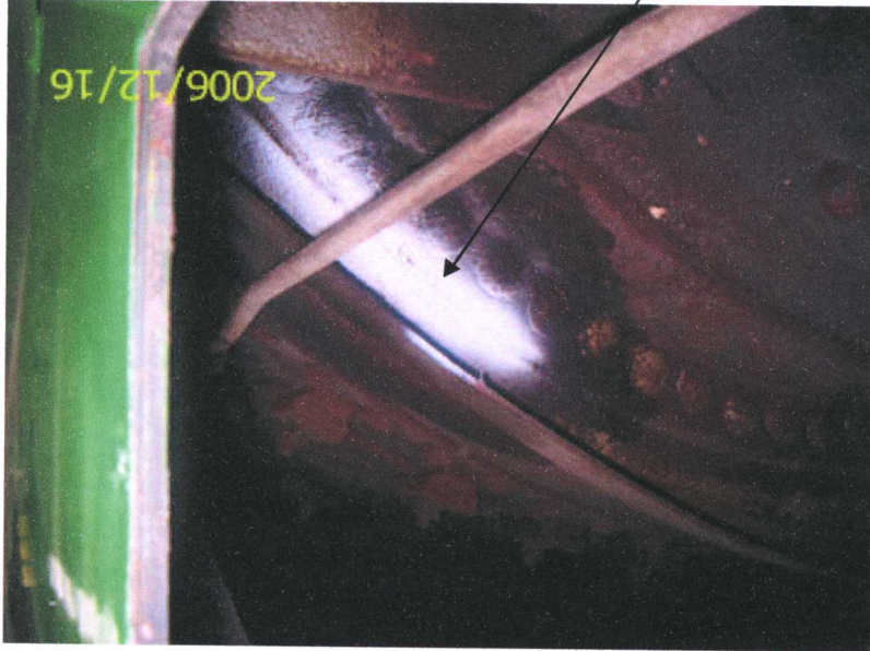
Photo 9 Barrel angle ring/ smokebox tubeplate RHS Location of leak on caulking
