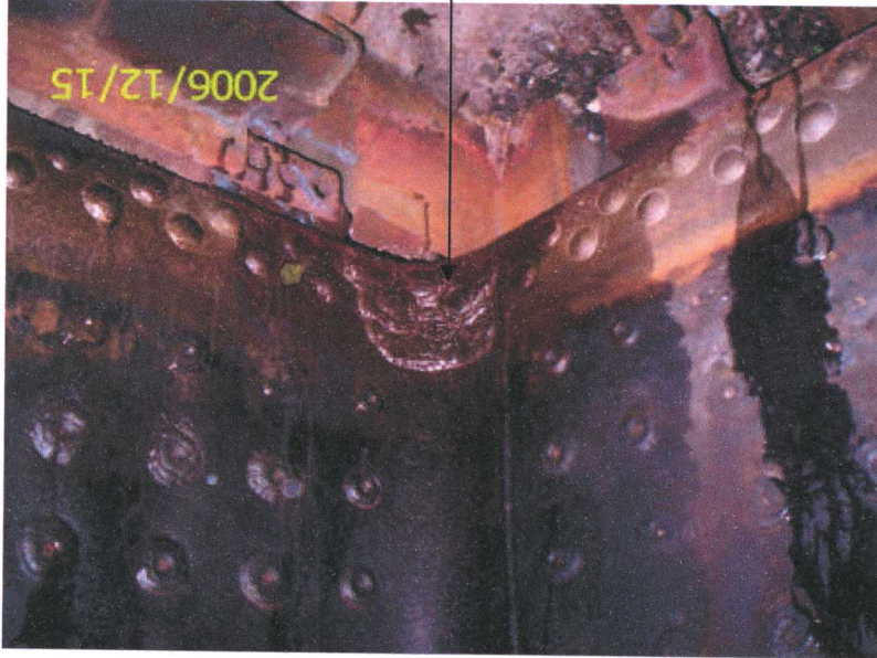
Photo 5. Old weld repair Firebox RH rear corner
