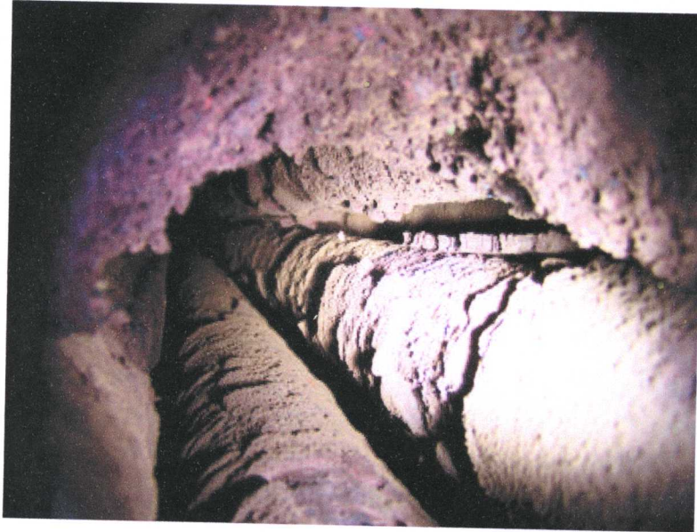
Heavy scale on boiler tubes
