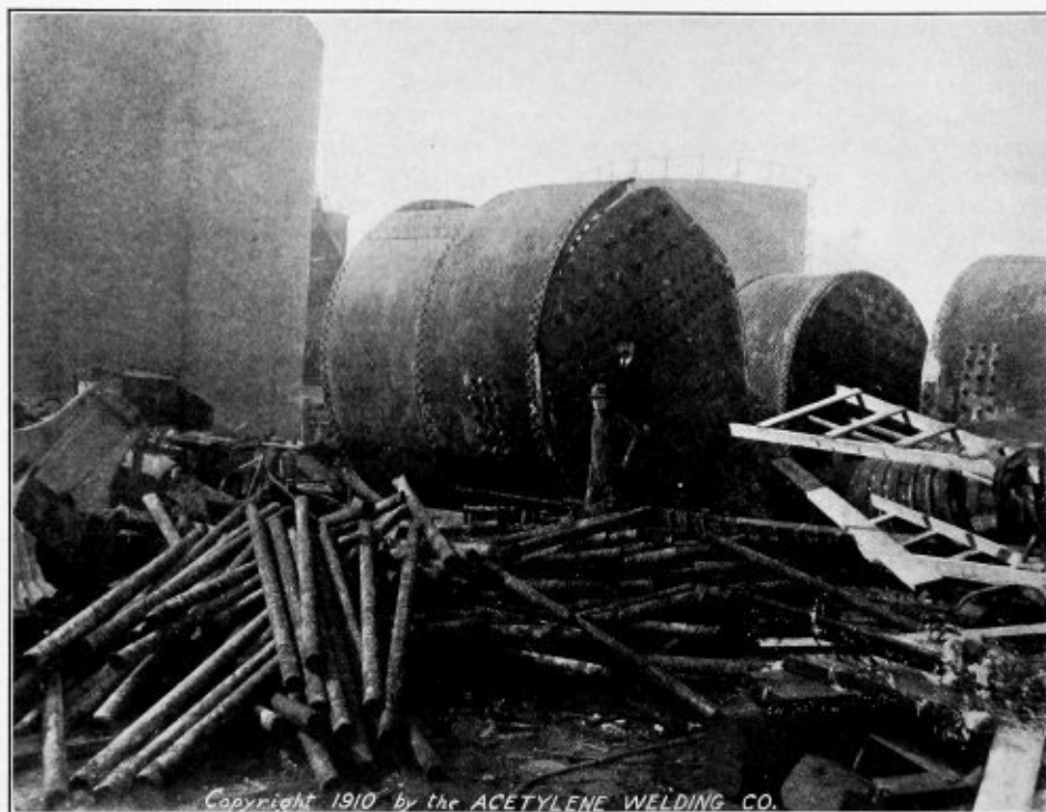
DEMOLITION OF FOUR SCOTCH MARINE BOILERS BY THE USE OF OXY-ACETYLENE CUTTING TORCHES.
