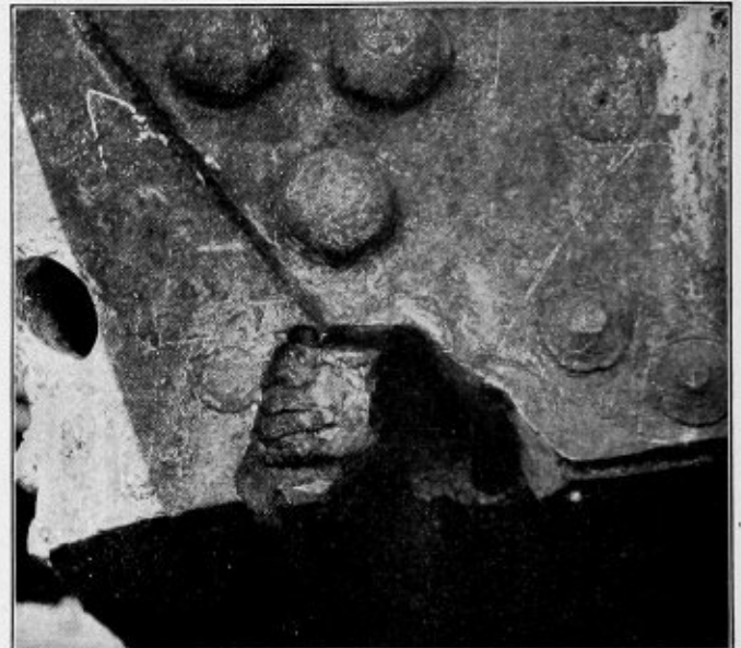
FIG. 2.—IT WAS NECESSARY TO REMOVE MORE OF THE DEFECTIVE MUD RING AFTER BEING PARTIALLY WELDED
