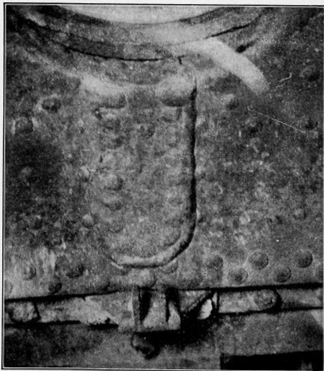
FIG. 5.—PATCH UNDER FIRE DOOR WITH EDGES WELDED INSTEAD OF CALKED
