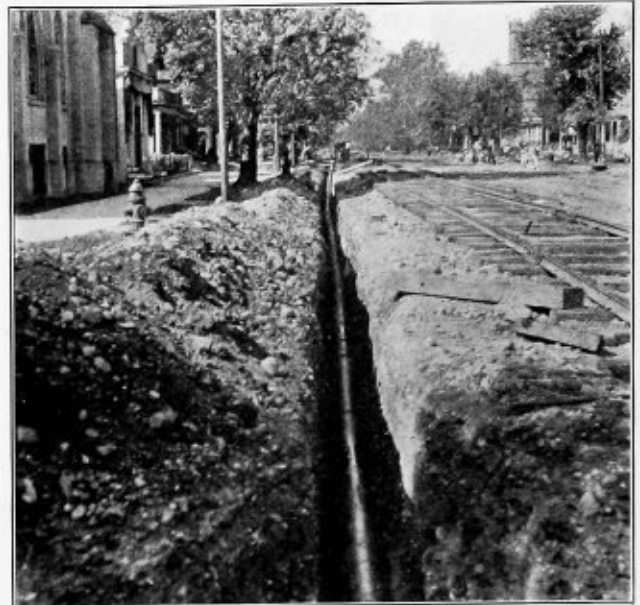
Fig. 2.—Twenty-Four Lengths of 10-Inch Pipe, Each 20 Feet Long, Welded Into One Section
