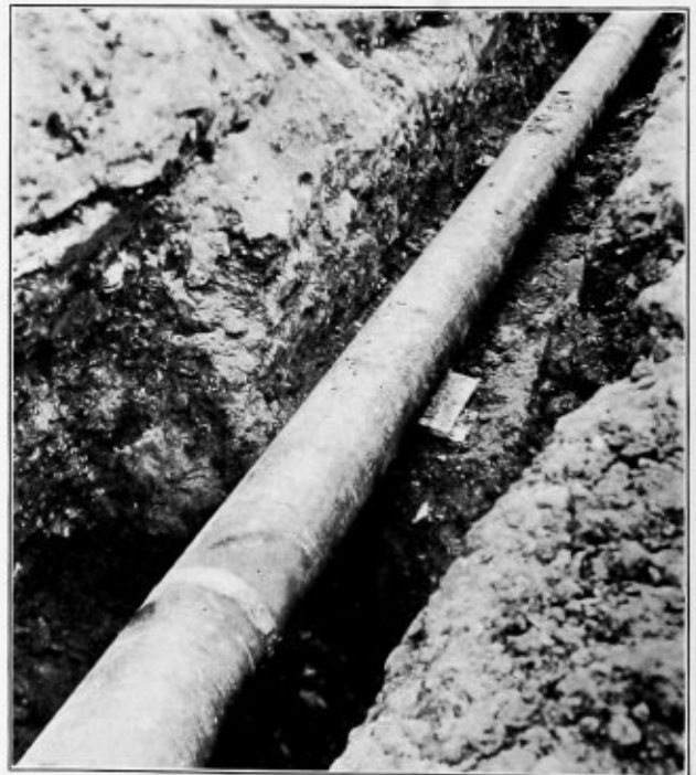
Fig. 3.—Welded Joint in 12-Inch Gas Main. Entire Joint Welded in the Trench
