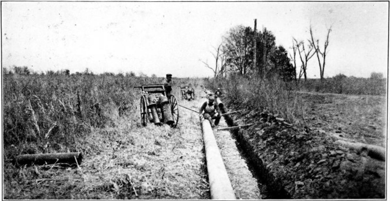
Fig. 4.—Method of Carrying Oxygen and Acetylene Cylinders through Rough Country for Welding Gas Mains
