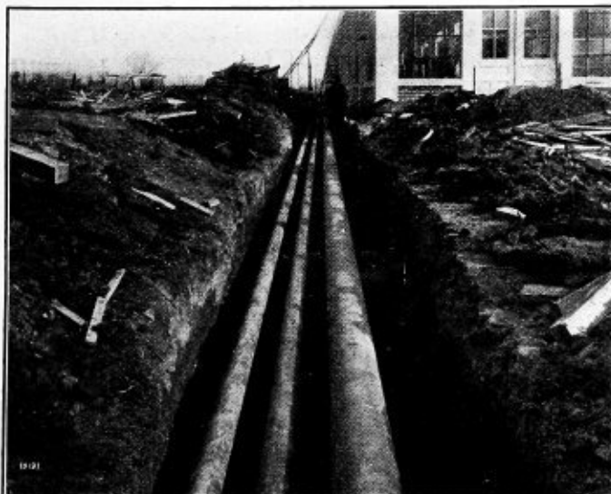
Fig. 3.—8-Inch and 4-Inch Pipe Lines
