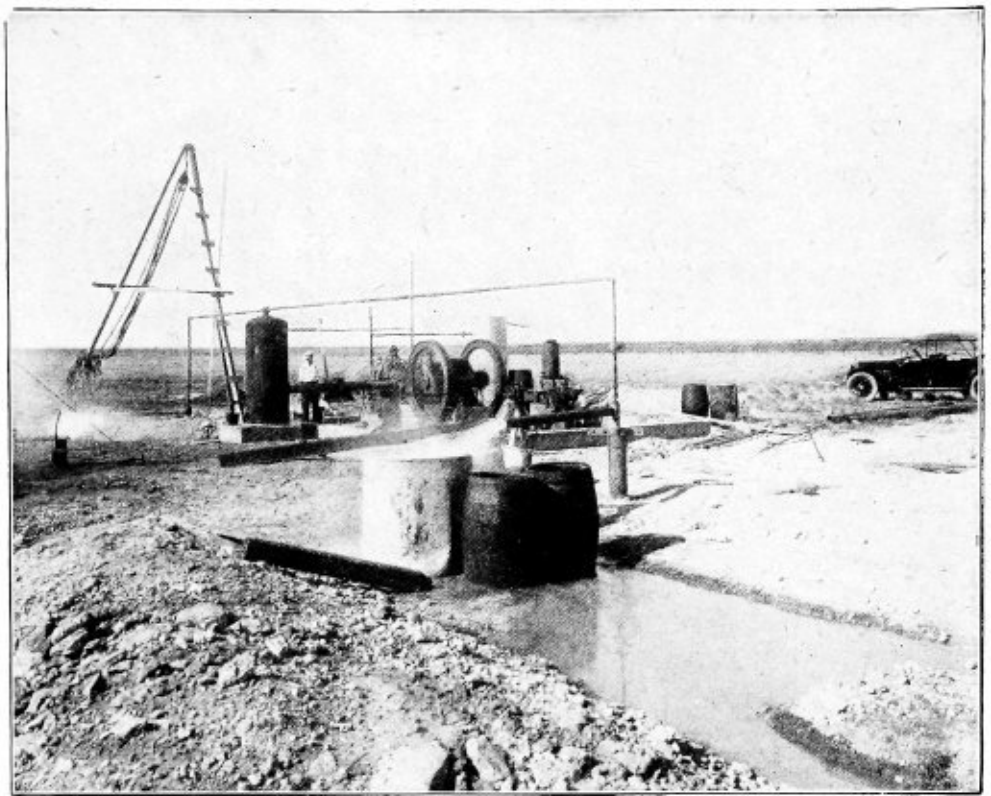
Class N-SO "Chicago Pneumatic" Compressor Pumping Wells on Texas Ranch
