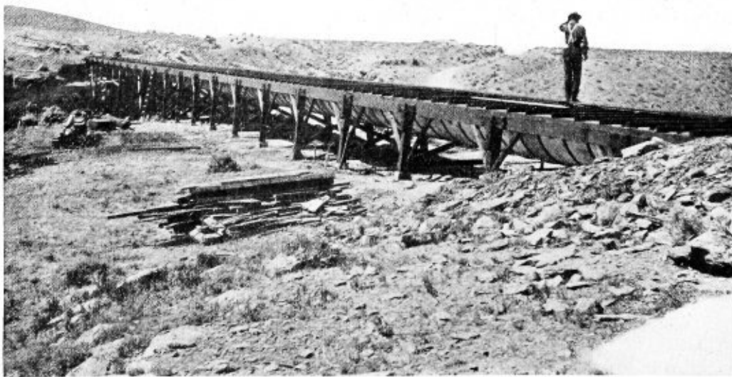
Fig. 3.—Hess Armico Metal Flume of Redlands Irrigation & Power Company, Grand Junction, Col.
