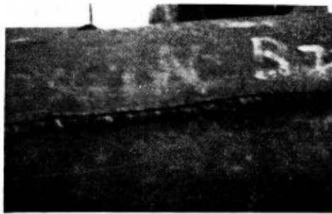
Fig. 5.—Tank No. 1. Enlarged View of Part of Bursted Seam
