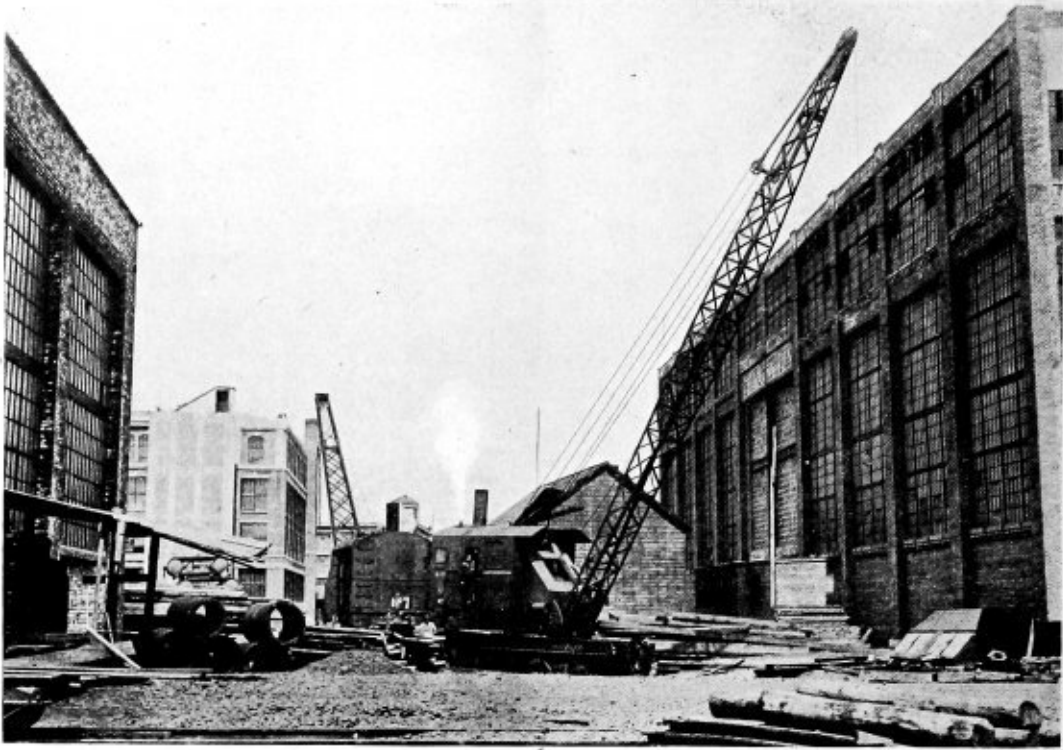
Fig. 5.—Locomotive Cranes Are Utilized to Handle Material in the Yard and Supply the Laying-Out Floor
