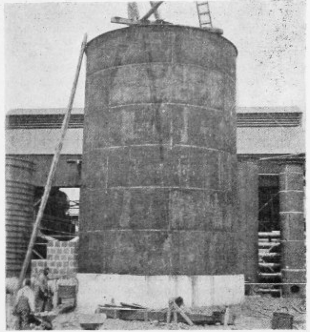
Gas Tank 22 Feet in Diameter, 30 Feet High, Welded Throughout by Acetylene Process
