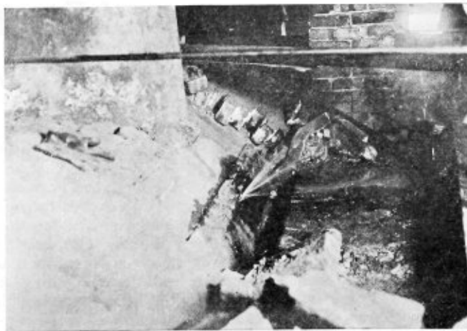
Water Shown Issuing from a Lap Seam Crack
