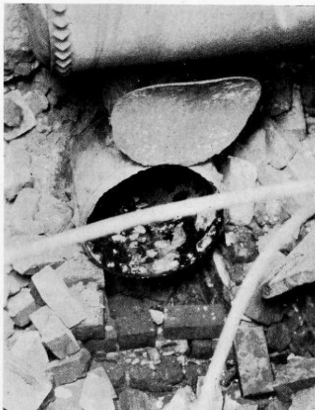
Failure of Blind Mud Drumhead on Horizontal Tubular Boiler
