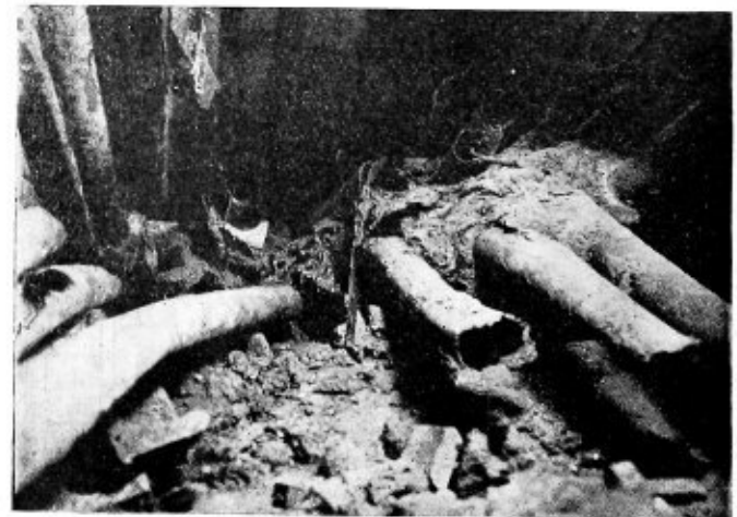
Fig. 2.—Damage Caused by Firing Up an Empty Watertube Boiler
