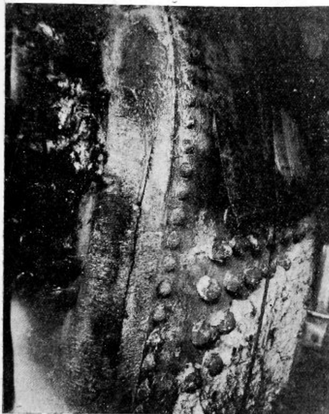
Fig. 3.—Fatal Crack Occurred in a Welded Repair Job
