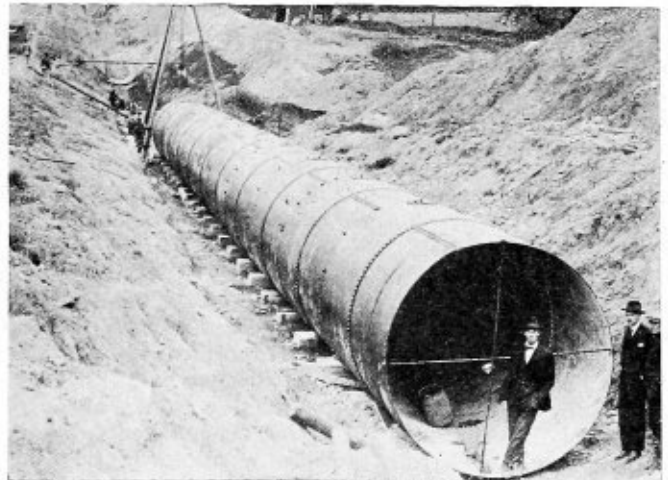
(Keystone View Co., N. Y.) Sections of Pipe Assembled at the Catskill Aqueduct Which is Used to Supply Water for all Purposes to the People of New York
