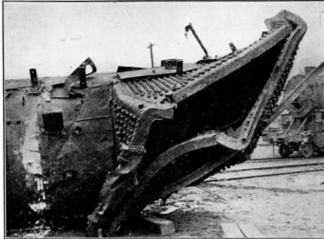
Fig. 1.—Back End of Boiler After Crown Sheet Failure
