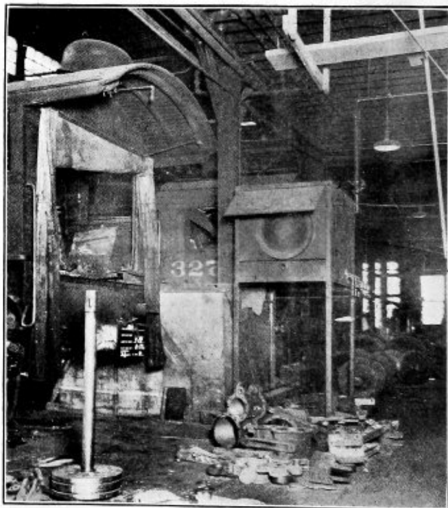
Unit heater installed in New York Central locomotive repair shop
