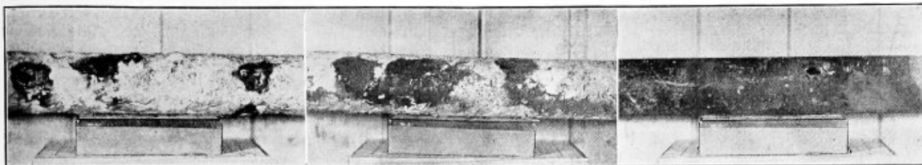
Three views of pitted and corroded tubes
