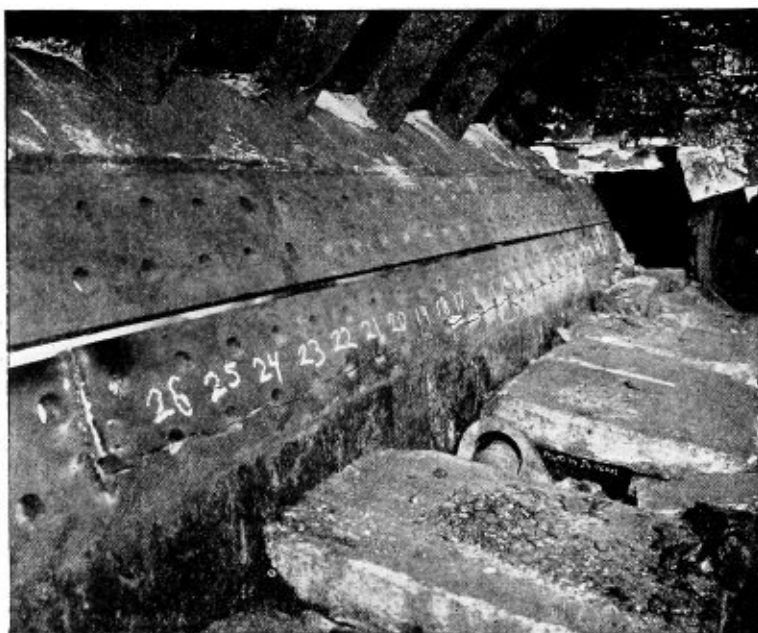
Fig. 8.—Outside of embrittled drum in 500 horsepower boiler
