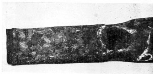
Fig. 17—Superheater flues sometimes cause trouble
