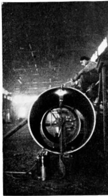
Fig. 4.—Preheating arrangement tried in preheating out V of longitudinal seams. Note how seam was tilted to facilitate building up of weld reinforcement
