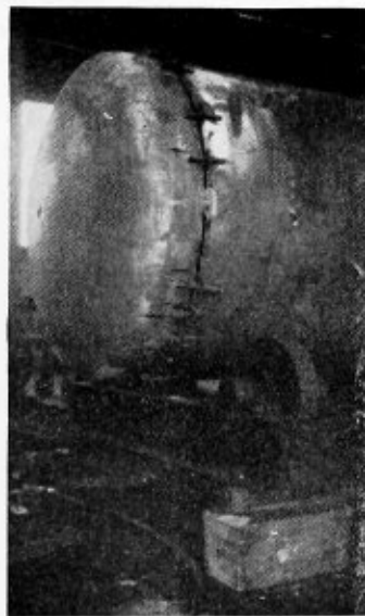
Fig. 6.—Method of securing desired spacing and alinement of girth seams. Note tack weld
