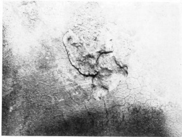
Section of plate showing surface defects caused by a deposit of foreign matter
