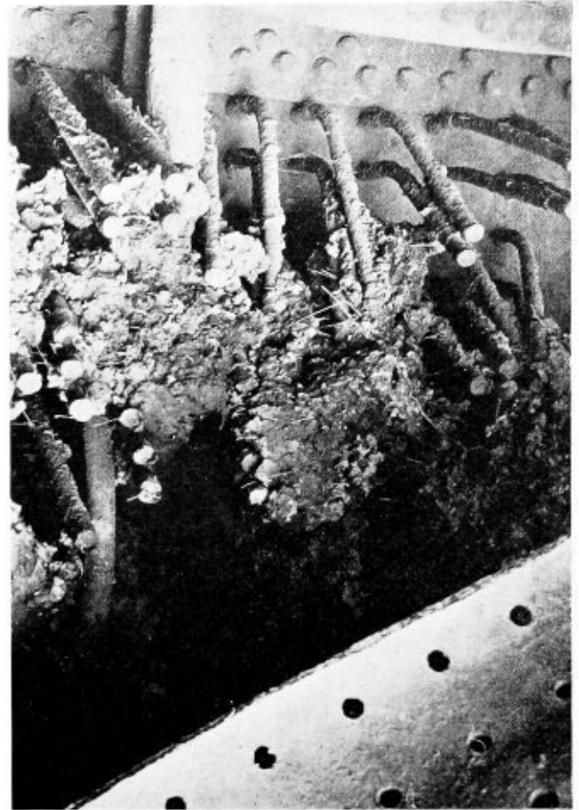
Fig. 4.—Where a side sheet seam failed for its entire length
