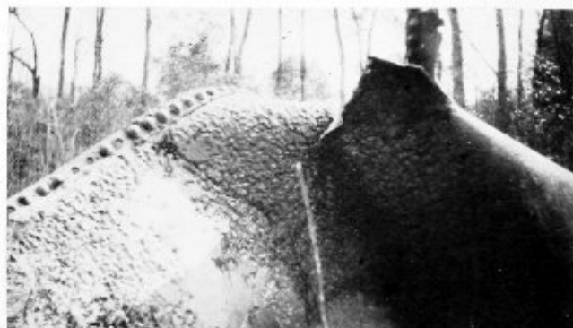
Ruptured boiler sheet
