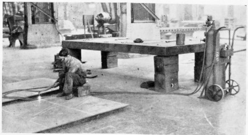
A section of the shop for laying out and cutting waist sheets
