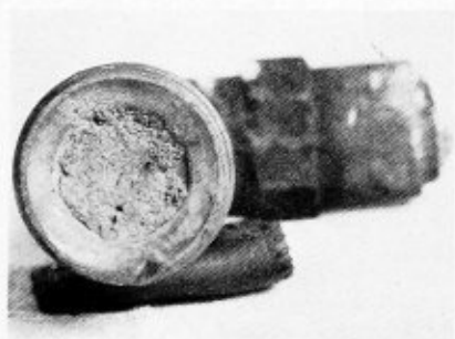
Fig. 4. (above) Water column, including steampipe and top boiler fitting. Fig. 5. (right) Water column connection, completely plugged by scale
