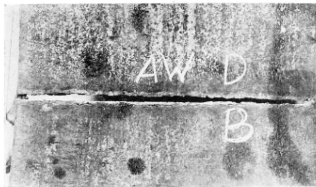
Fig. 3.—Welded butt joint of 1930 series after failure
