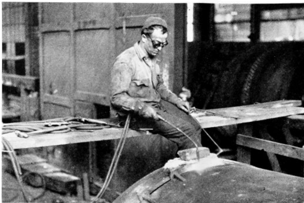
In the welding of pressure vessels tack-welds are supplemented by a series of wedge clamps
