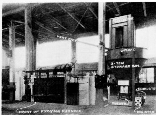
Fig. 2.—Storage bin, dust collector, feeding and burning equipment for one heavy forging furnace
