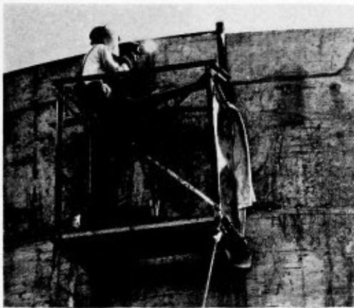
Fig. 4.—(Right) Lifting a top ring plate for 20,000 barrel tank. Fig. 5 (Above) Tack welds finished and welding operation started
