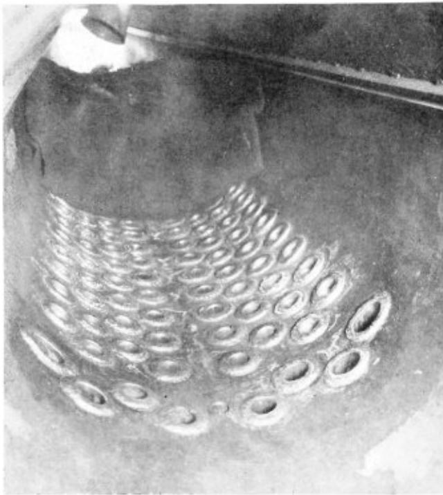
View inside 30-inch drum showing tubes welded to 4-inch drum shell
