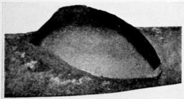
Tube failure which had serious consequences
