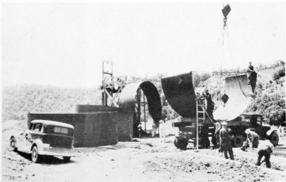
Section of penstock shipped to Norris Dam in semi-cylindrical sections, which were welded together into 20-foot lengths 20 feet in diameter
