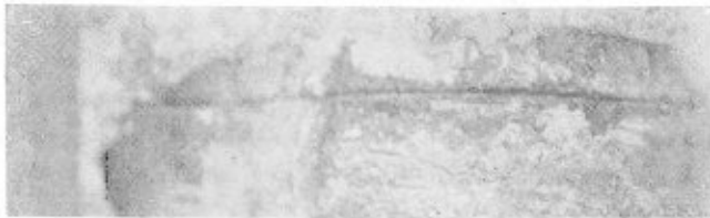
Fig. 3—Longitudinal crack in boiler barrel
