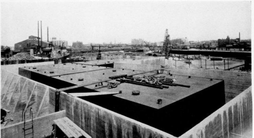
Fig. 2.—Three tanks completed ready for the installation of piping. All welding was done with the shielded-arc process
