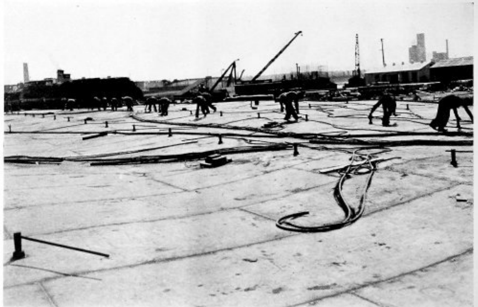
Hundreds of small plates were welded together to form the base plate for largest welded gas holder
