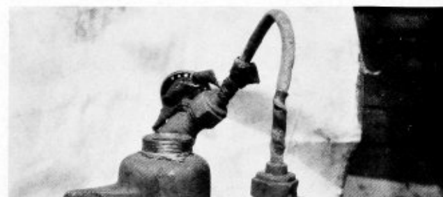
Fig. 8.—Twist in a water glass steam pipe
