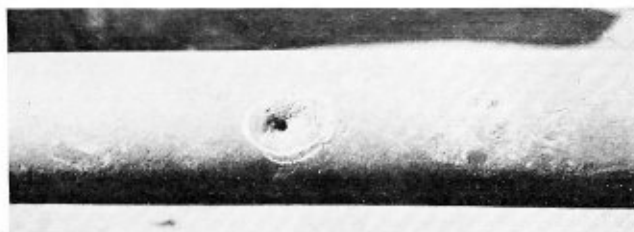
Fig. 5—Pitted superheater flue
