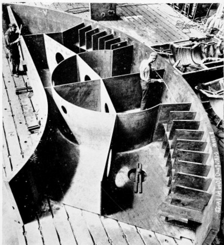
Fig. 5.—Fabrication of the upper end ring of the main tube section. Two welders are working on opposite sides simultaneously to batter distribute heating and cooling effects. Fig. 6.—(Right) Early stage in the construction of one section of the yoke horseshoe. Fig. 7.—(Bottom) Prime focus cage being moved into the annealing furnace
