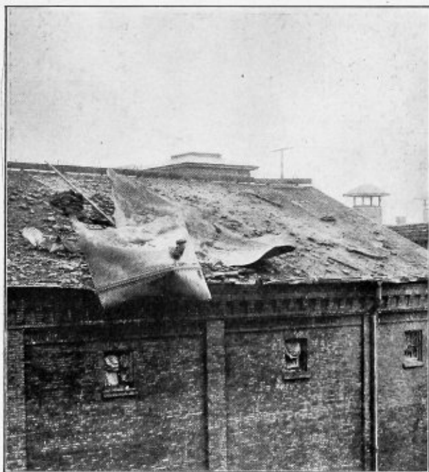
FIG. 3.—PORTION OF DRUM FOUND ON TOP OF FIVE-STORY BUILDING.
