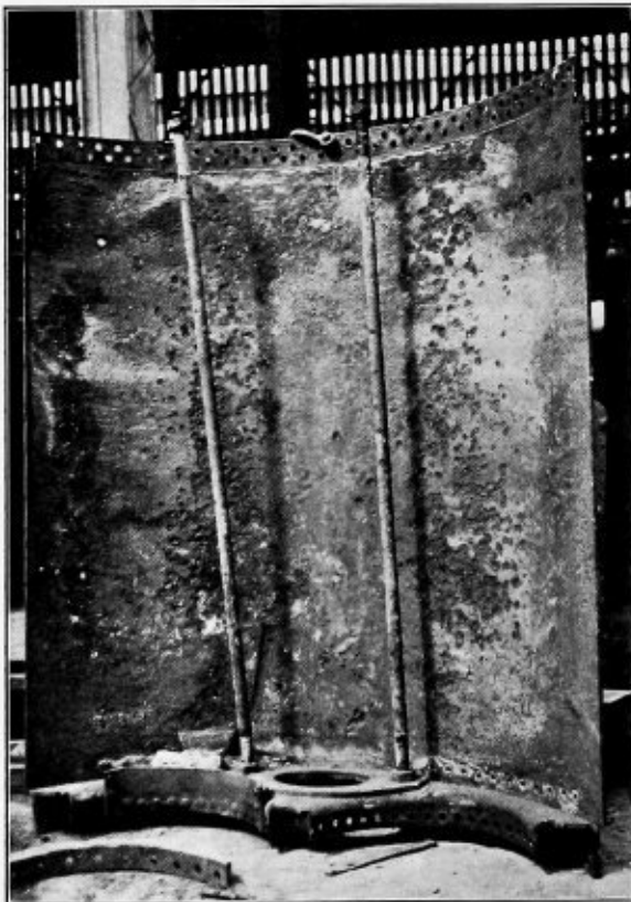
FIG. 2.—RESULT OF CORROSION AND PITTING IN THE LOWER PART OF THE BOILER SHELL.
